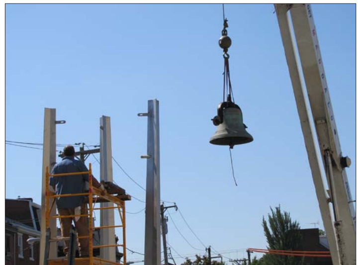
The Bell is lifted into the air by the crane. (Photos: T. Siwak)
