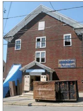
The original St. Michael's Ukrainian Catholic Church on West Center Street in Shenandoah is in the process of being demolished. It has not been used regularly as a worship site since 1908 with the exception of the early 1980s when Divine Liturgies were celebrated there due to a fire that destroyed the second church building of the parish. (Photo: Andy Matsko)
