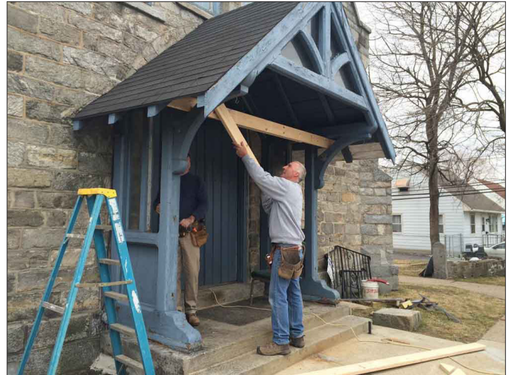
Original gate portico dating to 1819, that was moved to become a portico for the Church entrance being sured up. The portico is being moved to provide of ADA access to the Church. The portico will once again be used as a gate entrance from the parking lot through the cemetery garden path.
