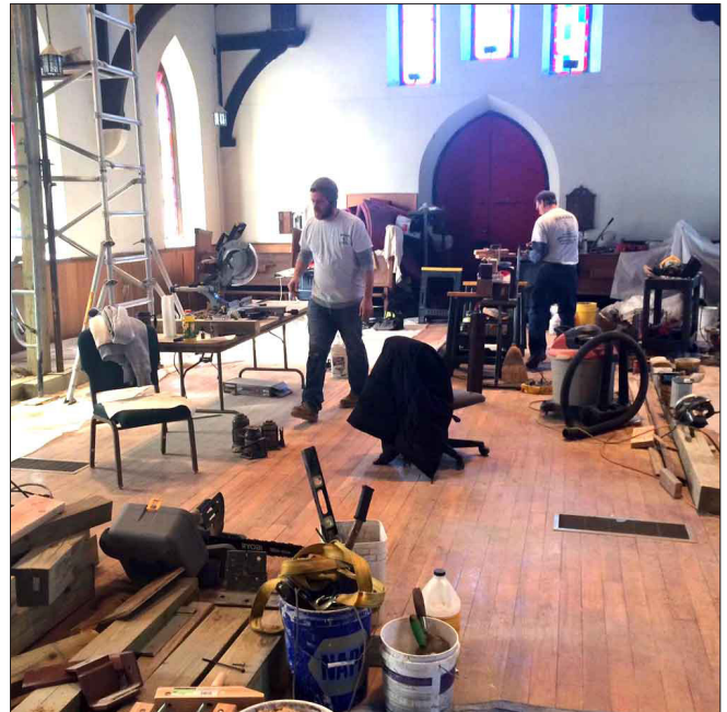
Kyle Rhoads and his Father Bill Rhoads working on the hammer beam renovations and replacements.
